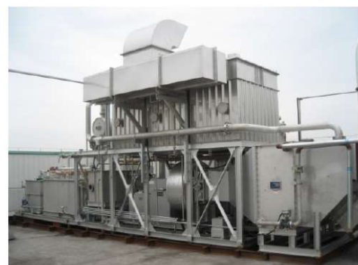
VOC recovery equipment
