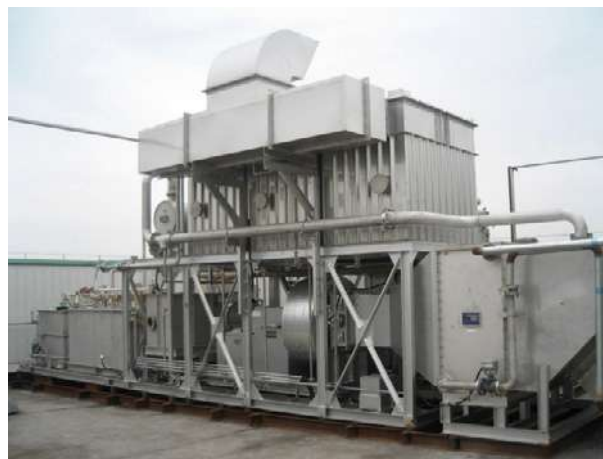
VOC recovery equipment
