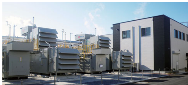
Gas cogeneration facilities at Japan Exlan Co., Ltd.
