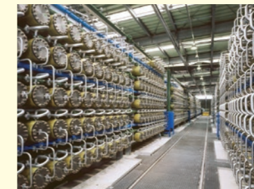
Seawater desalination plants
