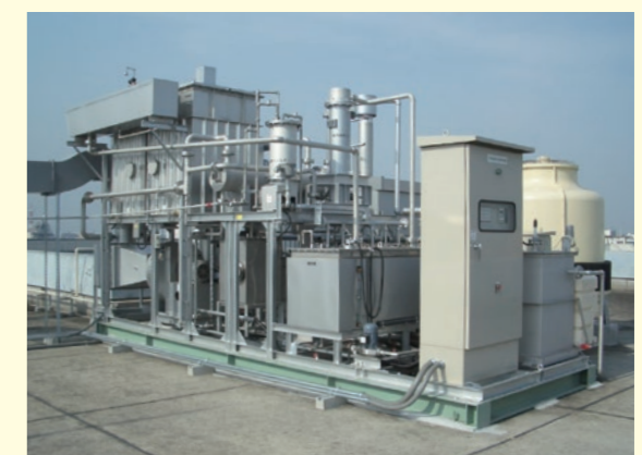
VOC recovery equipment
