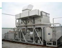
VOC recovery equipment
