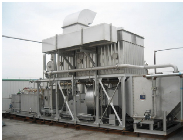
VOC recovery equipment
