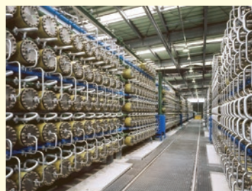
Seawater desalination plants
