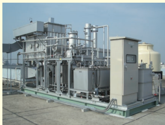
VOC recovery equipment
